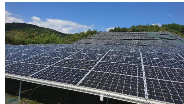
Photo: Awa Solar Power Plant in Tokushima
